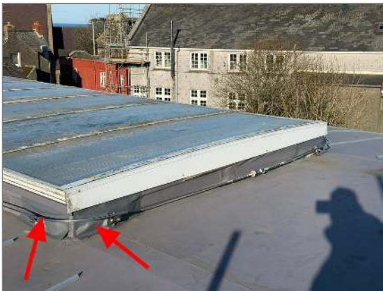
Photo - 12 Poor flashing detail around raised perspex sky lights.
