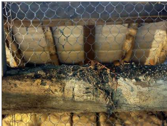
Photo - 18 Active wood boring infestation and softening of the timbers
