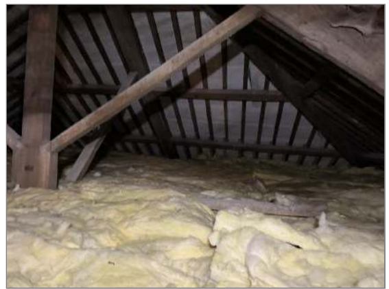
Photo - 17 Well insulated roof space which prevents access
