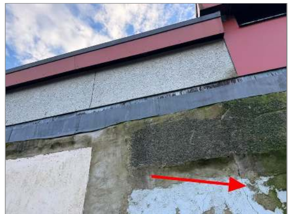
Photo - 14 Rendered section to extension and lead detail to join. Crack in render to join.
