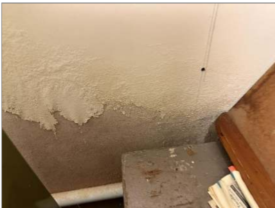
Photo - 26 Obvious damp issues to room off clerk office
