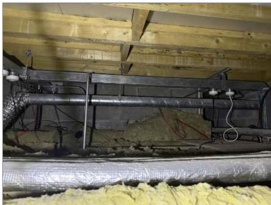
Photo - 23 Voids over WC's
