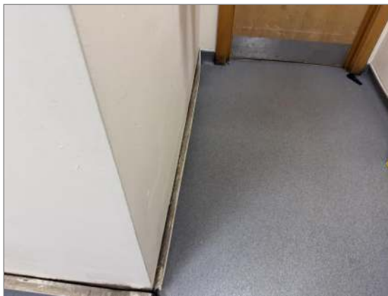
Photo - 27 Loose floor covering in the kitchen
