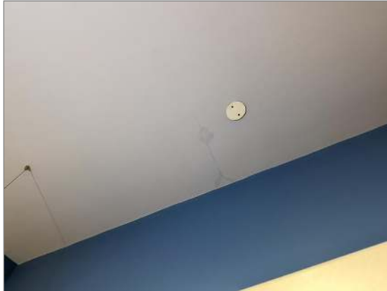
Photo - 21 Stains to tapestry ceiling
