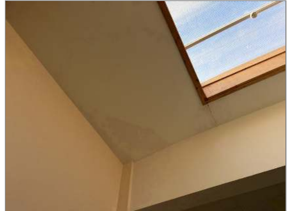
Photo - 22 Stains to domed roof
