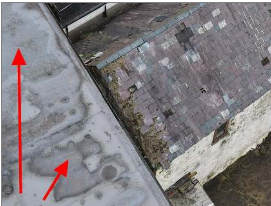
Photo - 6 Ponding to flat roof.
