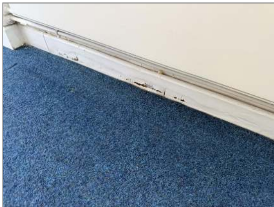
Photo - 28 Cuboidal cracking to skirting - indicating potential dry rot
