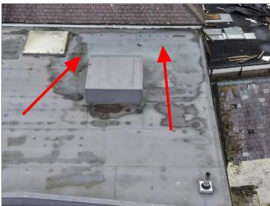
Photo - 8 Ponding to corner and around raised structure.
